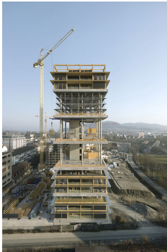
Figure 2. Holliger Tower competition, 4. Prize, Bern (with TEN architects, Neven Kostic structural designer).
