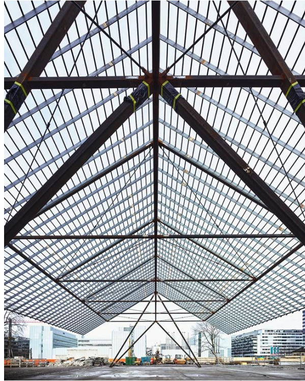
Figure 3. Koch Areal Zürich, Building site (with Krebs&Herde and Park Architects, Neven Kostic structural engineer)
