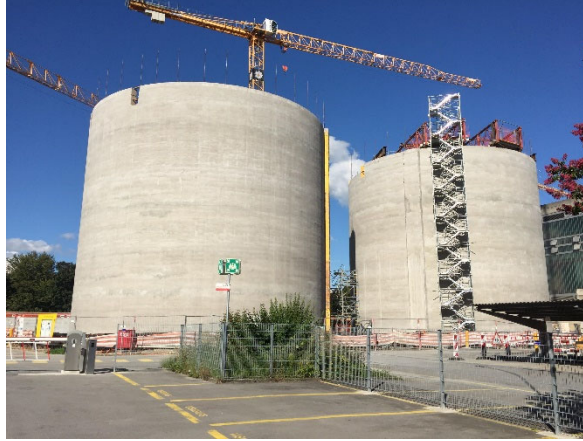
Figure 3. The new digestion silos of the Lausanne Water Treatment Station in Lausanne, Switzerland (Synaxis SA Lausanne civil engineers).
