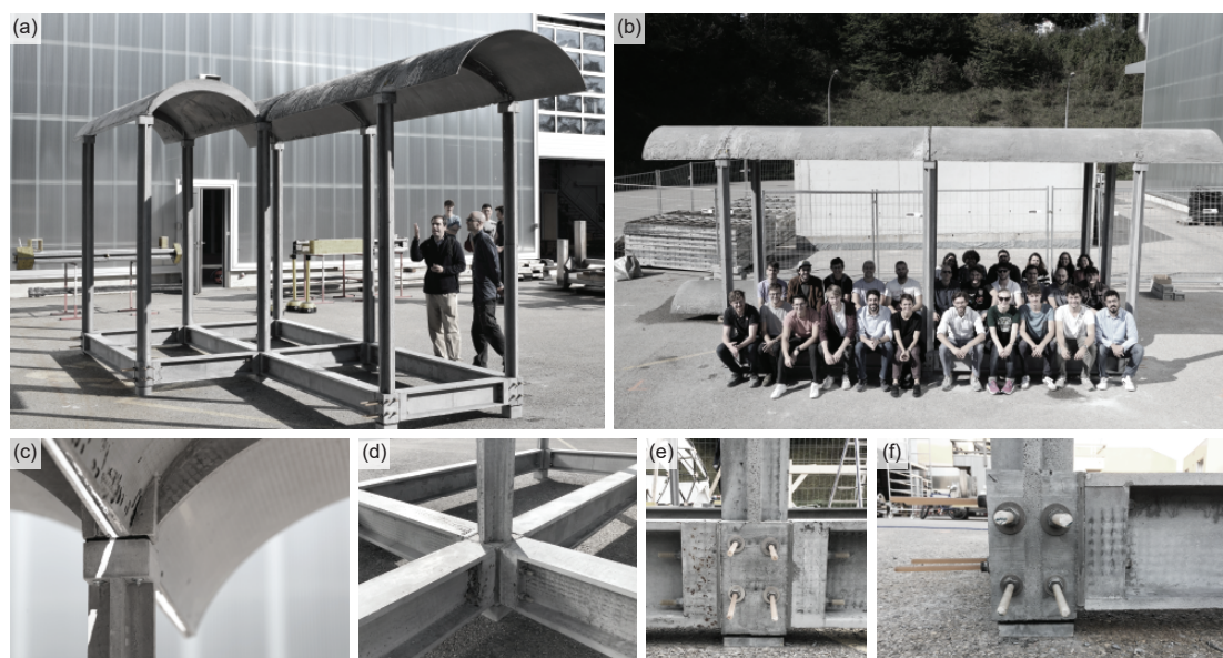
Figure 4.11: Final structure: (a) three modules; (b) construction staff; (c) column-head connection; (d-f) connections of the base frame.
