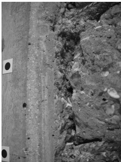
a) Gravel specimen (Crack level)
