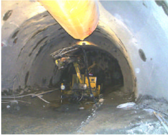
Figure 18. Picture of the metallic fibre reinforced sprayed concrete excavation support at the southern portal of the Gotthard base tunnel
